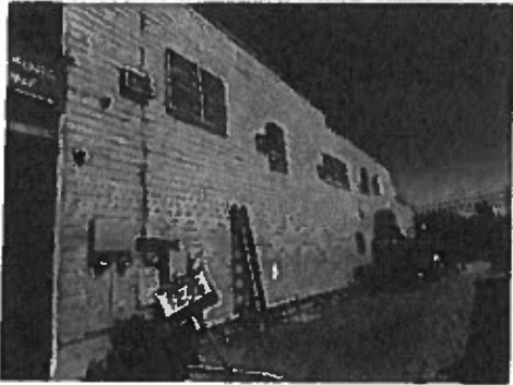
note mounted swamp cooler
