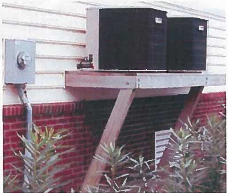
Figure 4-11 Elevated Outdoor Utilities
