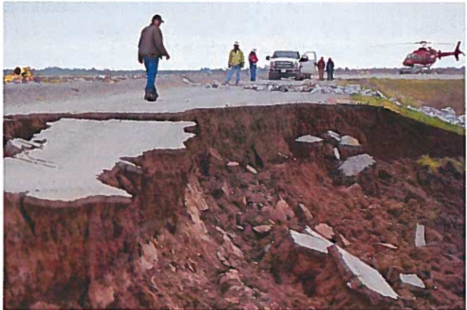
Figure 4-1: Tyler Island Levee Failure
